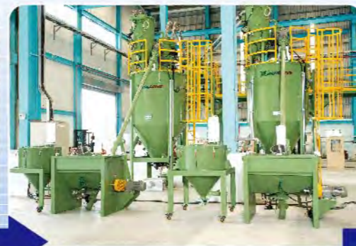
▲ C. 螺旋輸送至大儲料桶 SCREW CONVEYOR TO STORAGE SILO
